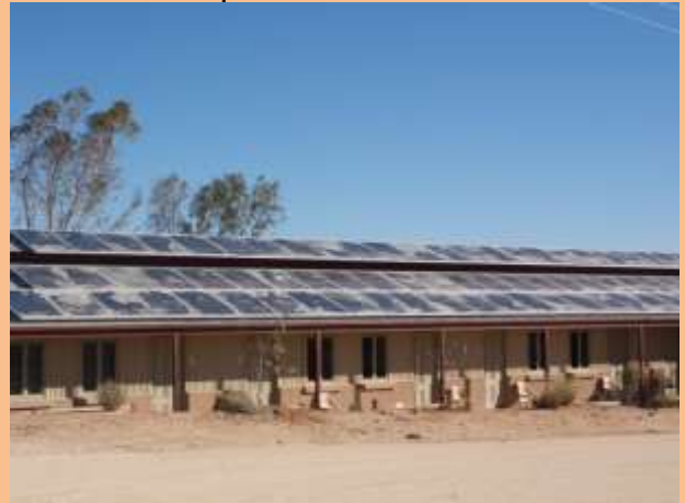
Solar Panels Innamincka Hotel. (Photograph K Buckley)
